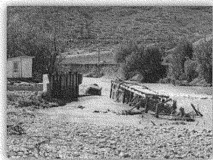
Figure 2 - Destroyed ditch company diversion and headworks
