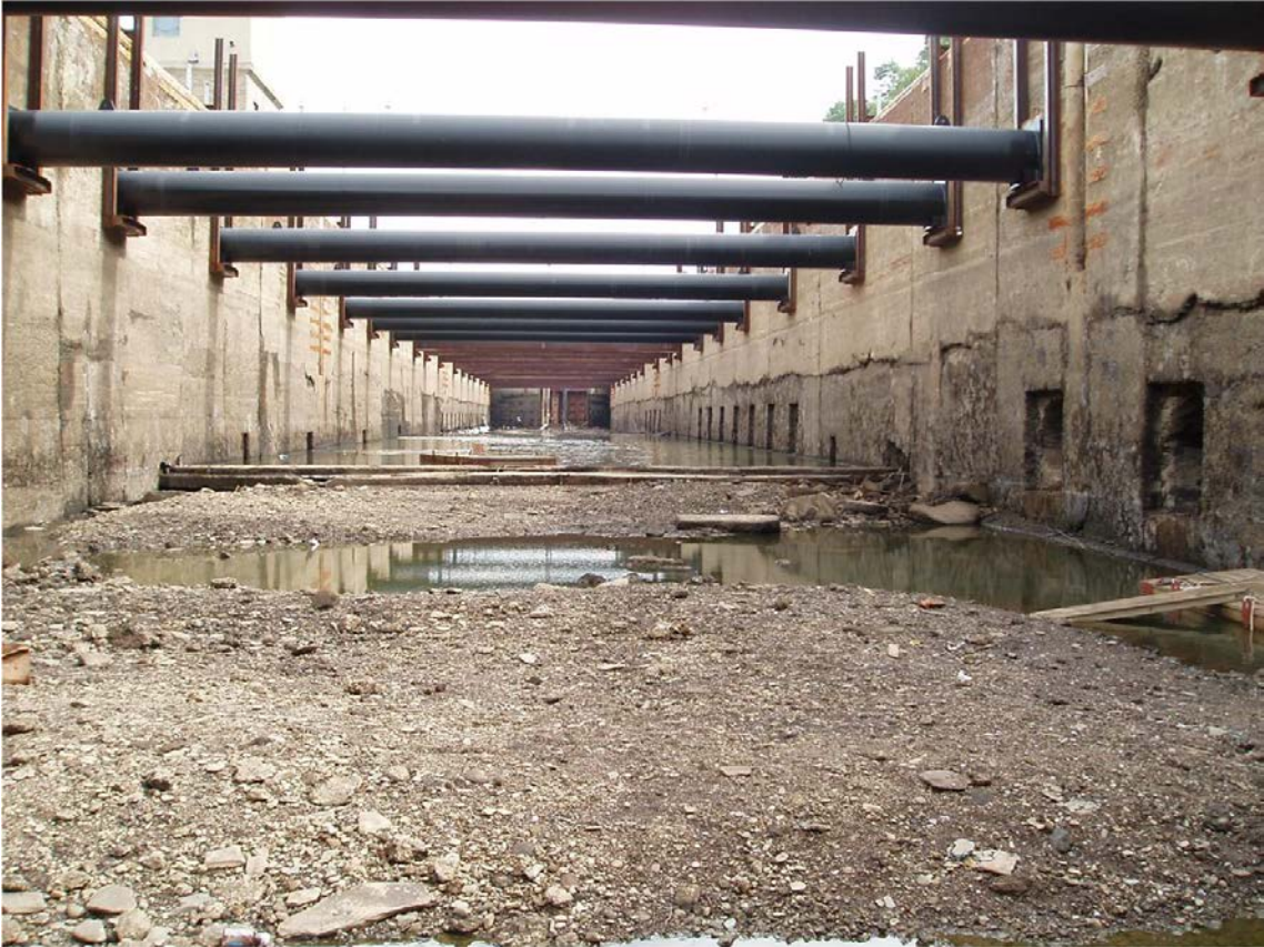
Figure 4 - Elizabeth Lock dewatered revealing its deteriorated condition
